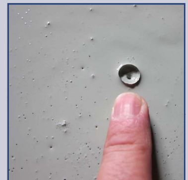
PINHOLES AND A POPPED BUBBLE REVEALING THE CRATER AND A PINHOLE
