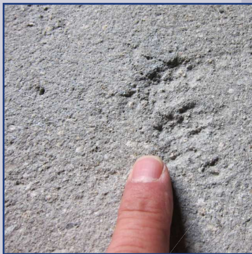
SUBSTRATE IMPERFECTIONS LEAD TO PINHOLES AND BUBBLES
